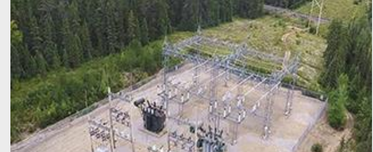
SUBSTATION, LA VERENDRYE, CANADA
