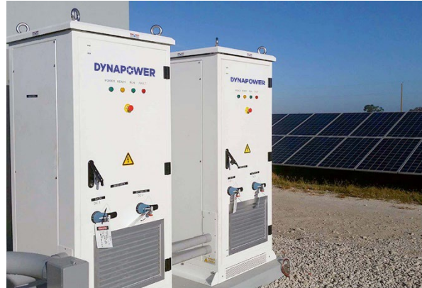
Dynapower DPS 500 DC- DC converters (image courtesy of Dynapower)
