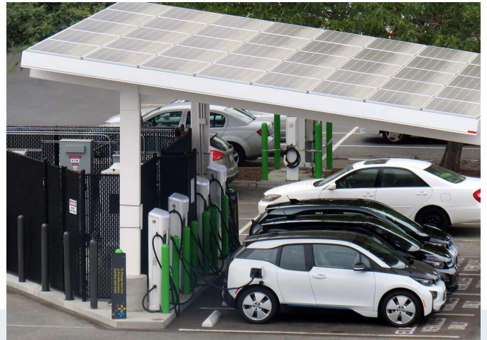
University of California San Diego (UCSD) combines the fastest electric vehicle charging, second-life EV batteries, and solar at the campus microgrid. Source: University of California San Diego
